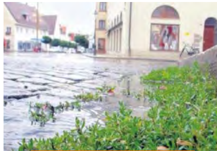
Problem: Clogged drains
